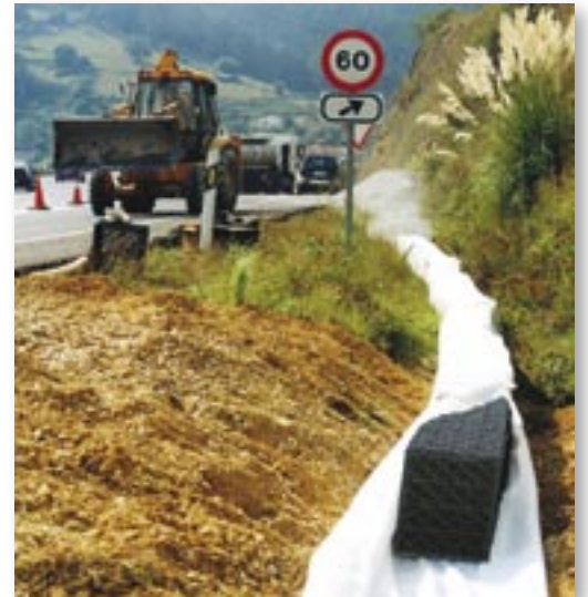
Installation of Atlantis Water Management solution into a highway in Valencia, Spain. Valencia is one of the most environmentally progressive communities in Europe.
