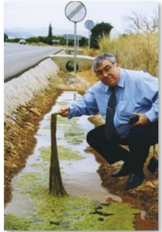
Poisonous green algae formed in open road drainage.
