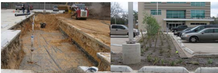
1. Digging out soil that was contaminated during construction and replaced with Bioswale mix 2. Completed Bioswale with plants placed on top of Atlantis Raintank
