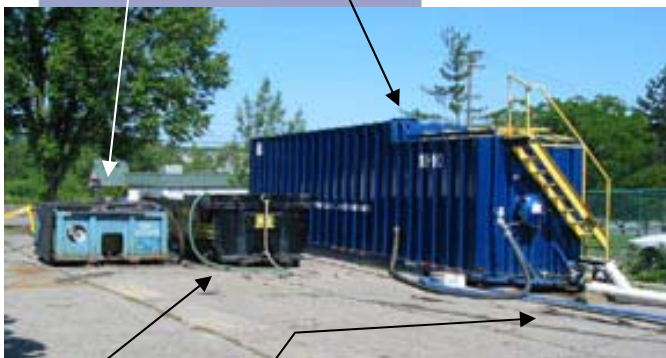
Settling Tank & Filter Polymer Clarification System
